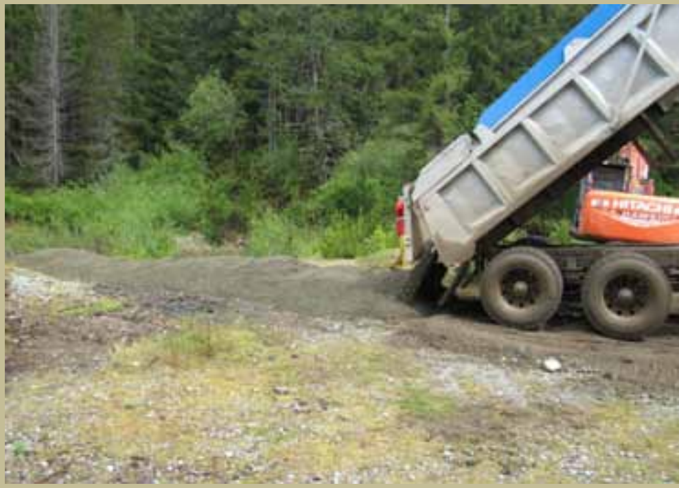
Sand was brought in and deposited along two ridges aligned east to west to provide a warm, south-facing nesting area for turtles.
