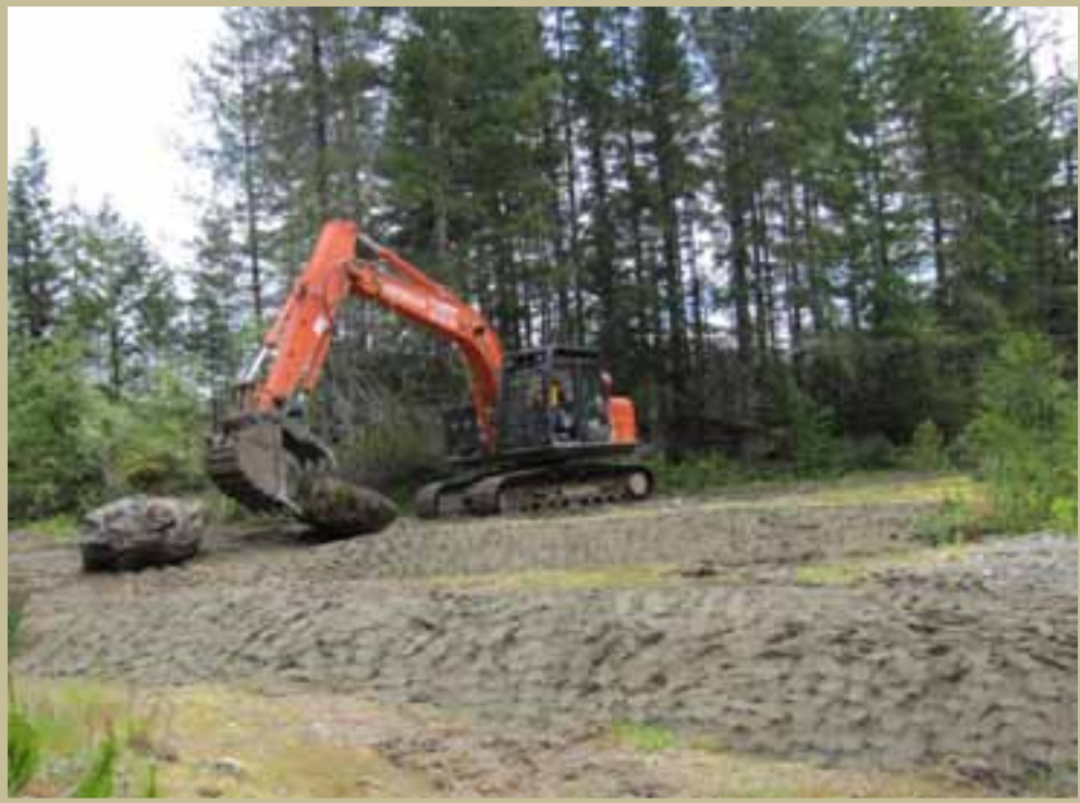
Creating a barrier of boulders to prevent unauthorized vehicle access to the site.
